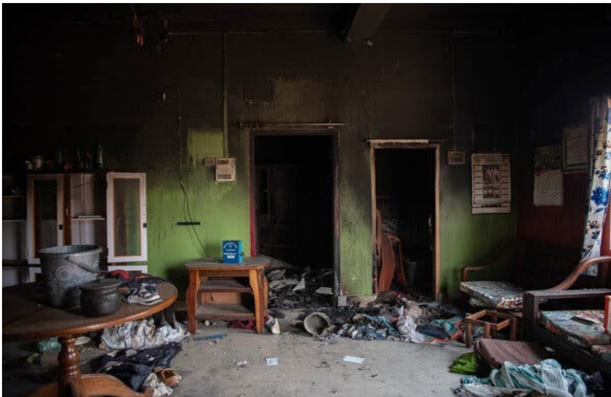
The damage done to a Kuki family's home in Imphal.
