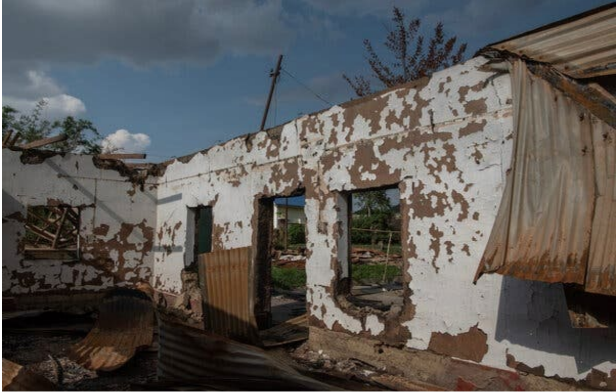
A house destroyed by arson.
